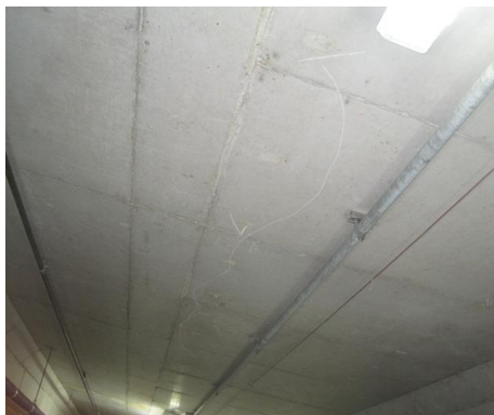
1련 Sta.0+52m 중균열(cw=0.2mm, L=4.0m)
